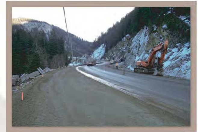
The existing shoulder in this segment west of the Rafter's Pullout will become part of the travelled portion of the widened highway in the future.
